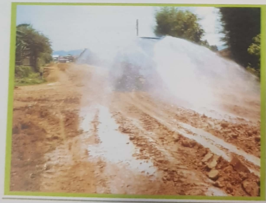
Figure No. 5 ORDINARY WATER MIX IN THE ROAD AFTER THE STAB-TECK APPLICATION
